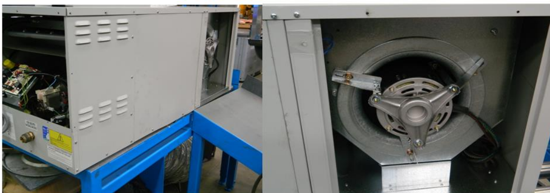
Photograph 13 and 14- Location of the fan motor
